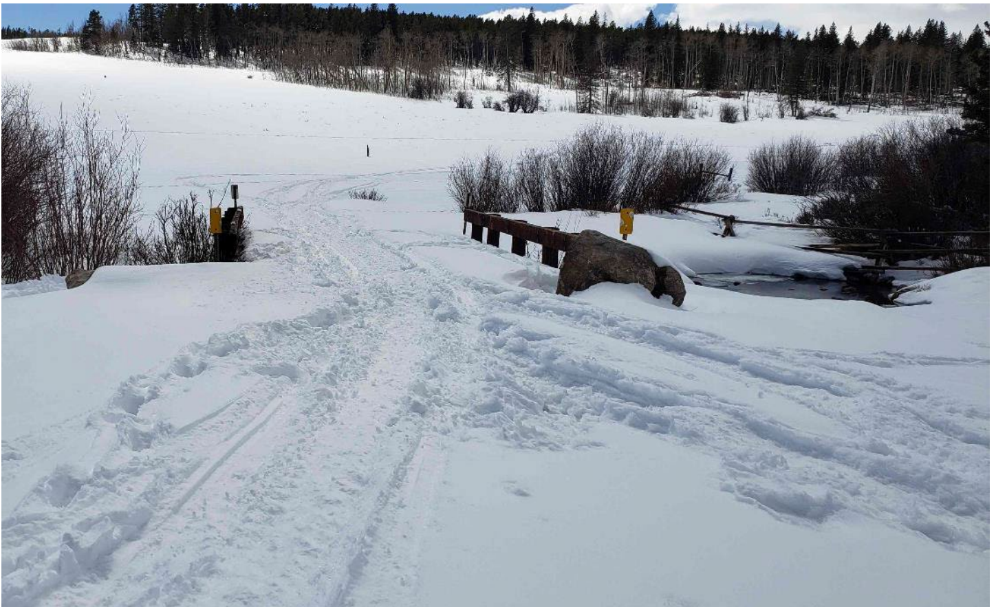
Hunter Creek Road, Johnson County, Wyoming. Photo credit: Wyoming State Engineers Office
